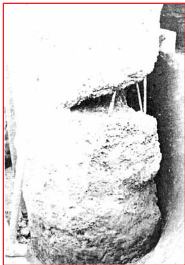
Fig. 18. Cavity in a pile due to soil ingress during the removal of the temporary casing. (Thorburn, S., 1977).
